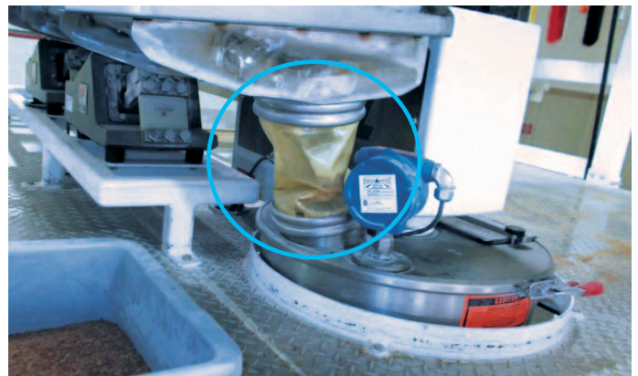
VIBRATORY SCREEN DISCHARGE TO AUGER FEEDER INLET - AFTER
